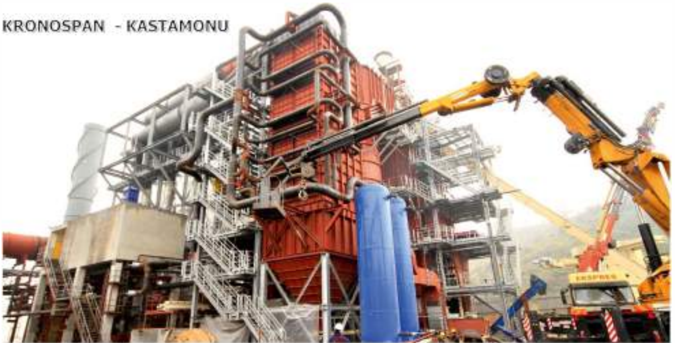
KRONOSPAN NEW WOOD PRESERVATION PLANT - KASTAMONU
